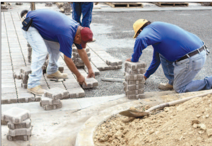
Paving units are placed on screeded No. 89 bedding layer over a No. 57 open-graded, crushed stone base. The joints between the units are filled with No. 89 material as well.
