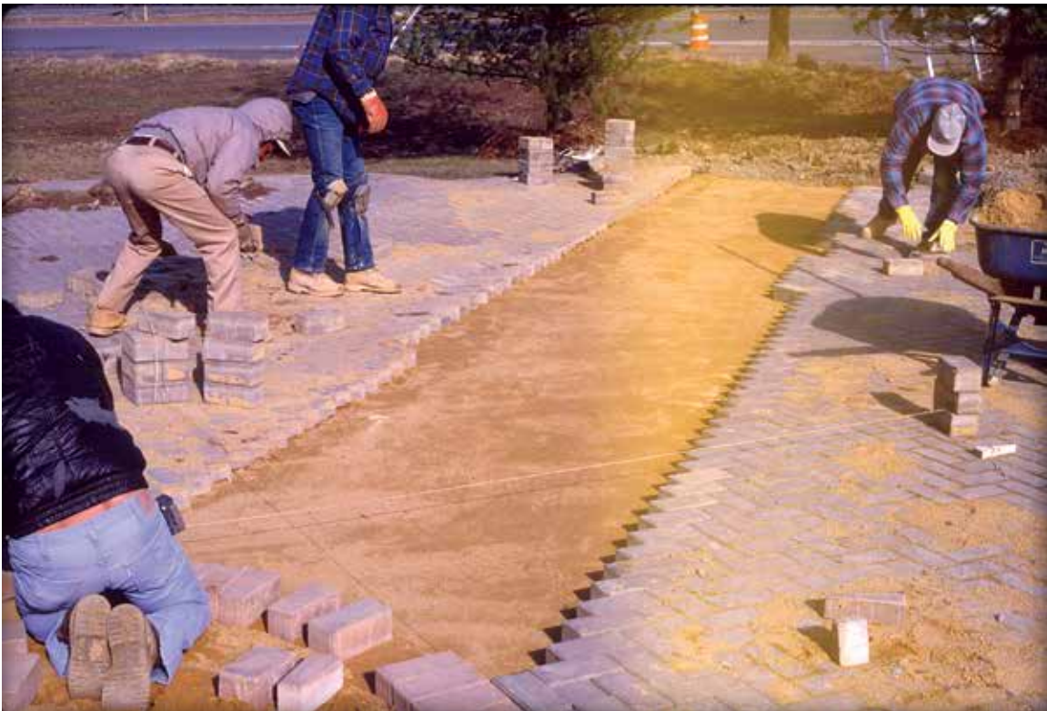
Figure 12. Screeded bedding sand. Note that a few courses of pavers are removed to create even sides for screeding. Installing temporary edge restraints prior to excavating is preferred practice.
