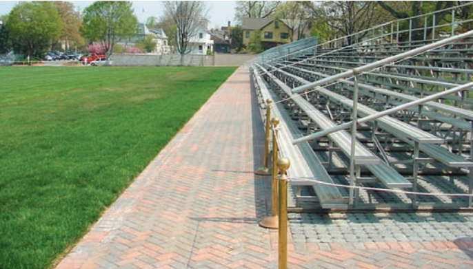
PICP under bleachers at the U.S. Naval Academy in Annapolis, MD provides structural support and on-site infiltration.
