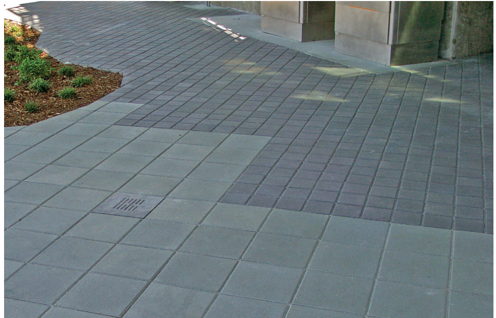
Shown: 6x6 Charcoal and 12x12 French Gray installed in a Stack Bond 45 degree pattern.
